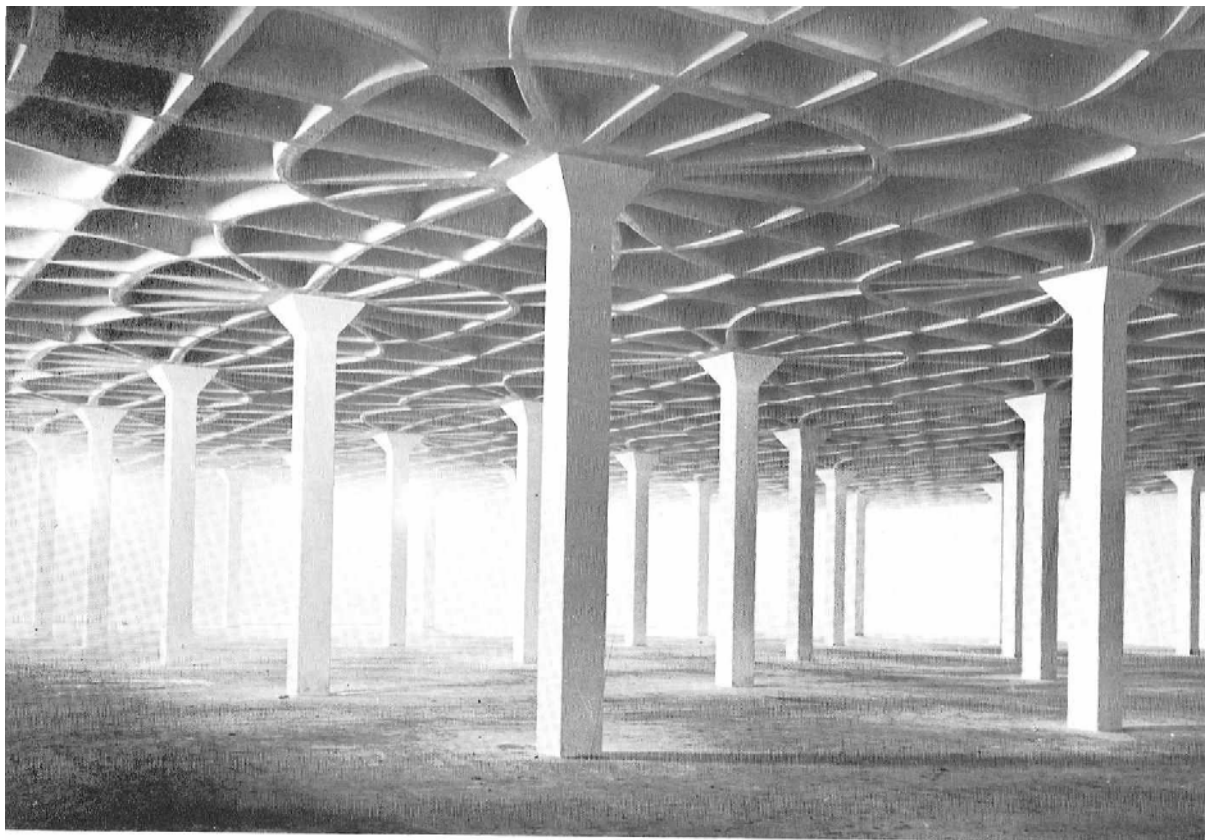
Fig. 49. Gatti Wool Factory, Rome: plan (left) and view of floor slabs with ribs following the isostatic lines of the principal bending moments.
